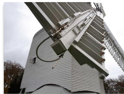
Sweep tip showing lightning conductor
